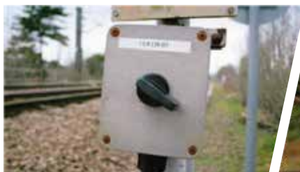
Example of a TOWS switch
