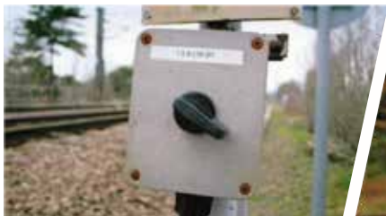
Example of a TOWS switch
